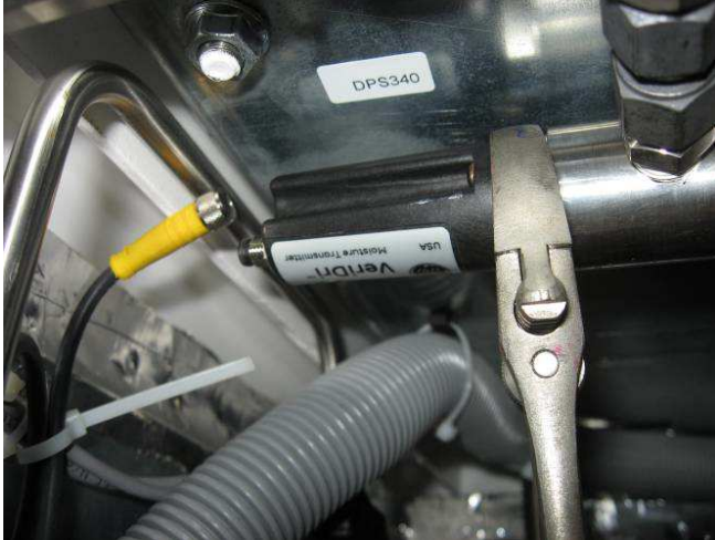
Figure 57 - Dew point sensor replacement
