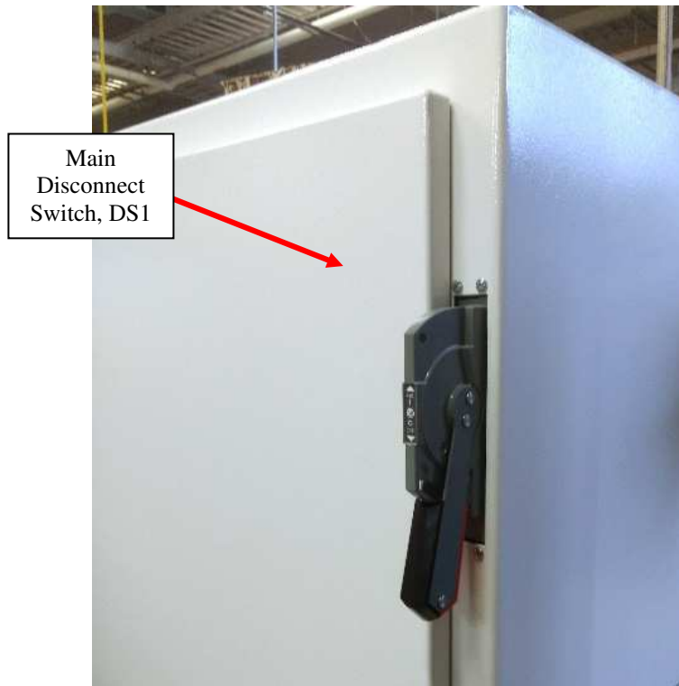
Figure 6 - C Series main disconnect switch, DS1
