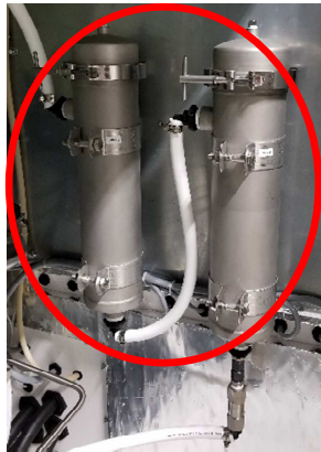
Figure 28 - Guard Bed Housing Assemblies Location
