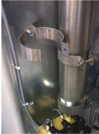
Figure 52 - Right Dryer Column
